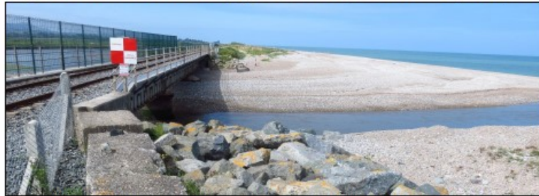
Railway bridge and shingle accumulations at the Breaches, looking north.
