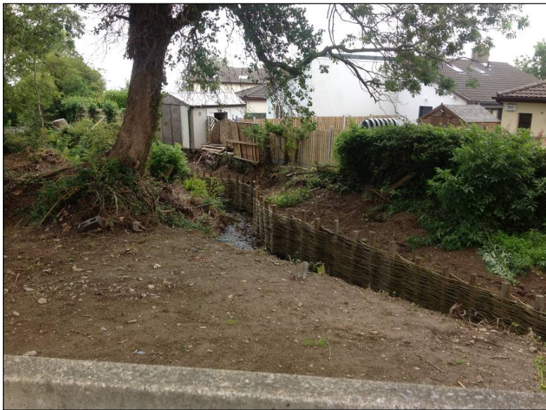
Plate 6. Damage to habitats, tree roots and vegetation during revetment works in 2020.
