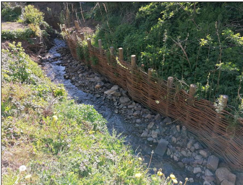
Plate 10. Willow revetment on the Kilruddery Deerpark Stream in St. Crispin's.
