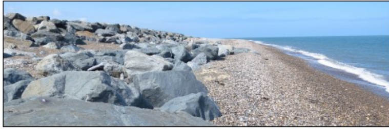
Shingle beach and coastal defences (greywacke boulders) at Six Mile Point, looking north.
