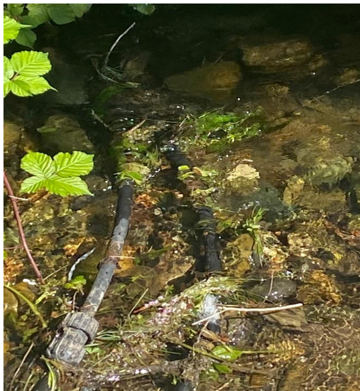
Leaking water pipes in the river.
