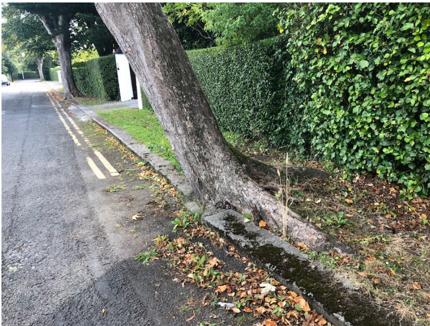
Fig. 33: View of tree causing damage to cast concrete kerb while being at risk of falling.
